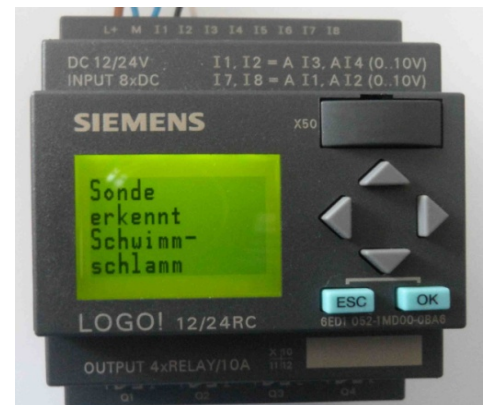
sonde has detected float sludge
