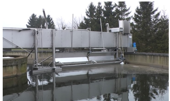
8. Hereafter the float sludge is underpassed again. After an adjustable time (e.g. 5 min.) the process starts new
