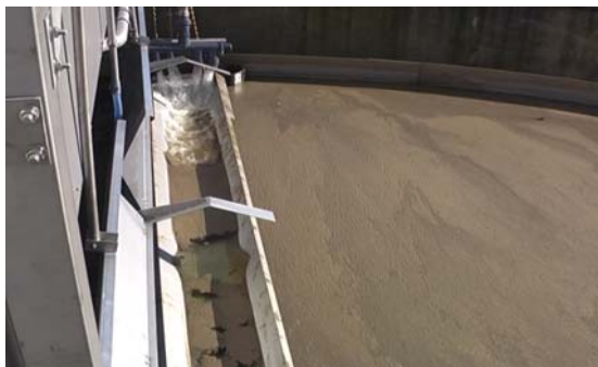
5. A drift stream delivers now the float sludge to the end and pushes it together
