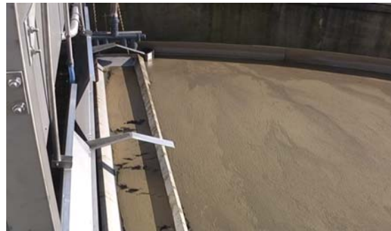
4. After this operation the sludge is separated in the thickening channel which forms now
