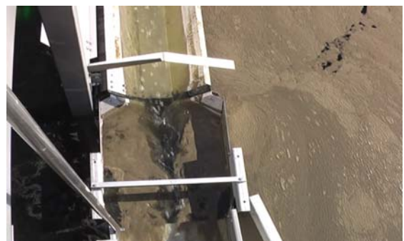
6. The excess and drift water flows at the other end of the supply and thickening channel down and back into the clarifier tank
