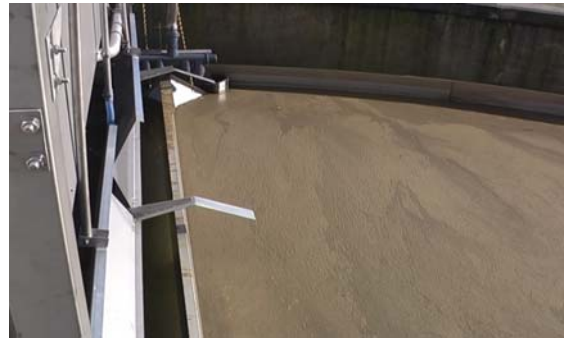
2. The float sludge is now underpassed by the paddling mechanism
